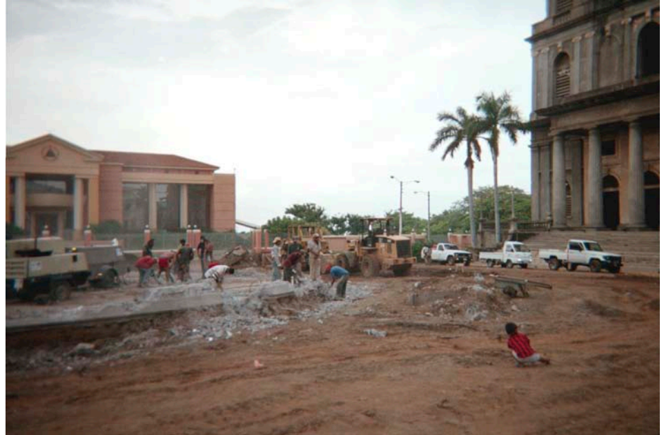
Crews demolish the fountain built by Arnoldo Alemán in what was once the Plaza of the Revolution. Readers who have visited Managua may recognize the Presidential Office on the left and the Old Cathedral on the right. Photo by Michael Radtke.
